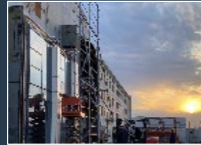
Curtain Wall Test Lab Shanghai, China
